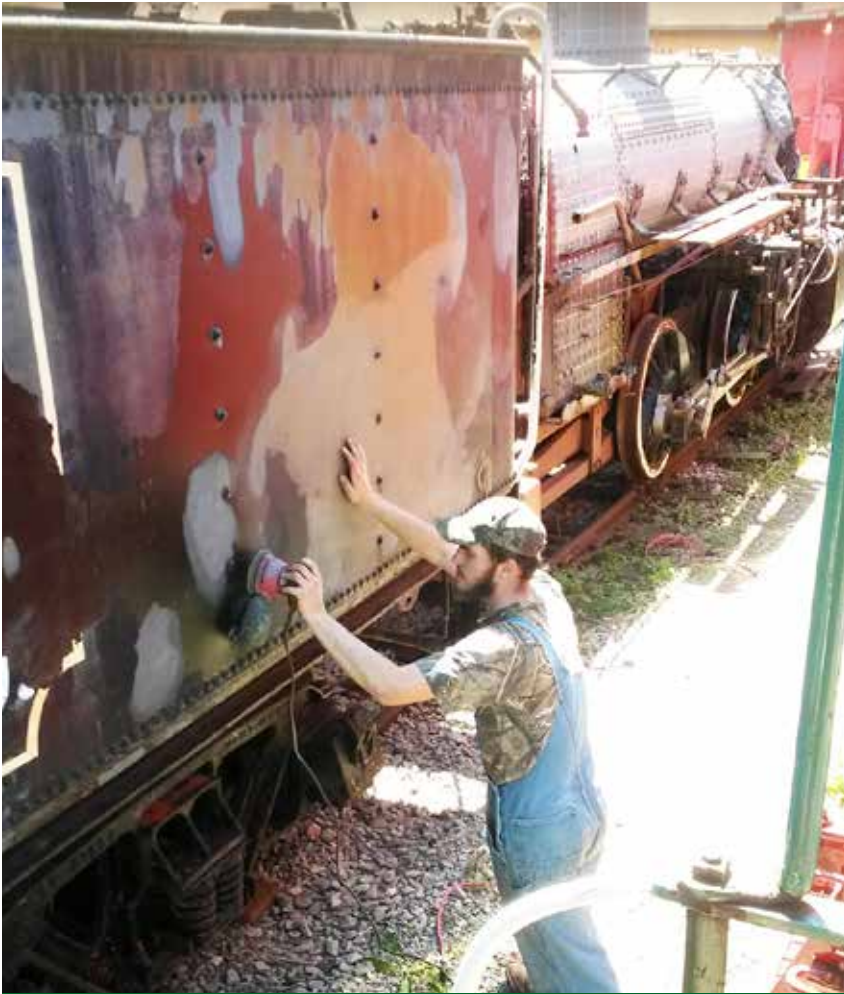
SANDING — Railroad volunteer Austin Croy sands the paint on the tender of No. 5 to get it ready for primer.
