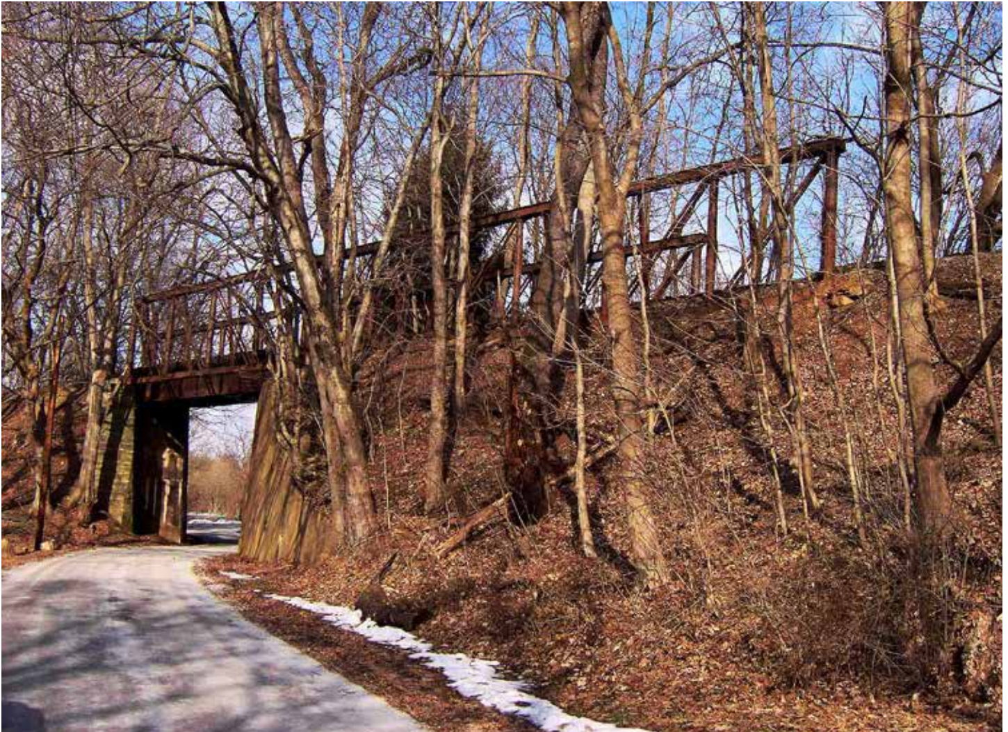
UNIQUE BRIDGE — Bridge No. 6, also known as the “Iron Bridge,” is made from a combination of second-hand iron and steel bridge parts supported by abutments of both fieldstone and concrete construction. The bridge was built in 1870 for the Pennsylvania Railroad and purchased used by the railroad.
